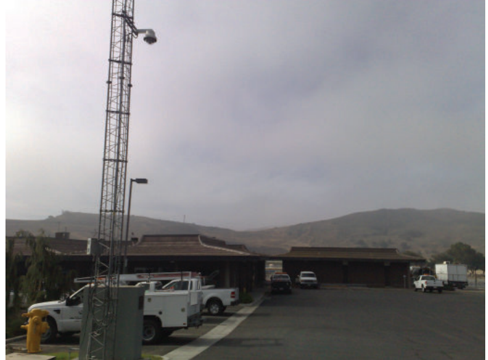
Outdoor IVC PTZ camera and wireless radio mounted on tower to monitor building and facility access and parking lot.
