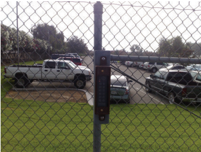
Isonas proximity card reader at facility gate.
